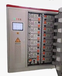
◆ GP Energy Storage
