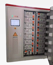
GP Energy Storage
